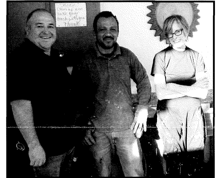
James Martinez and Ventura Herrera of CounterIntelligence installing the new GCC kitchen counter with GCA Board member Peggy Diggs. The kitchen remodel, led by Diggs, Barbara Seiler, and Shirley Hirsch, includes new granite countertops, sink, extended reach faucets, and re-painted cabinet doors. Mike Golino is also helping.
